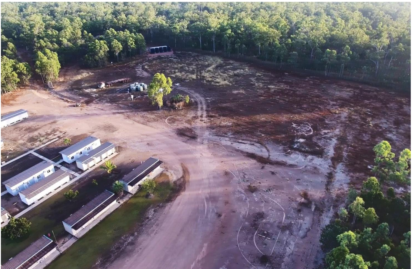
Figure 5: Cleared land for Bauxite Hills Mine new accommodation adjacent to the existing accommodation village
